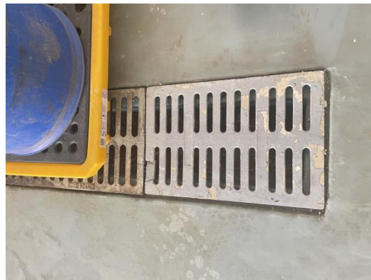
危废仓设无外漏通道的泄漏沟
